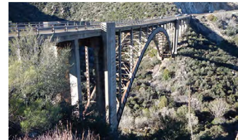
Steel arch bridge built in 1949; awarded the same year as "most beautiful steel arch bridge built in America" (Photographer: Scott Soliday)
