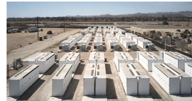
"Condor" stand-alone project, with lithium-ion batteries, California, USA
