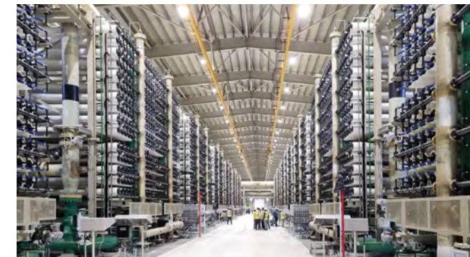
Yanbu 4 desalination plant, Saudi Arabia
