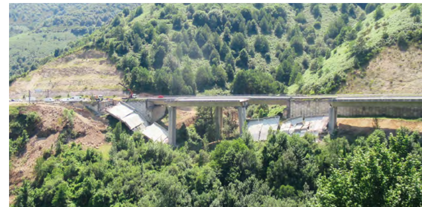
Collapse of Spans 1 and 3 of the Castro viaduct, direction A Coruña, Spain
