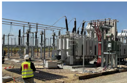
Electrical substation of the Los Alcores solar park, Seville
